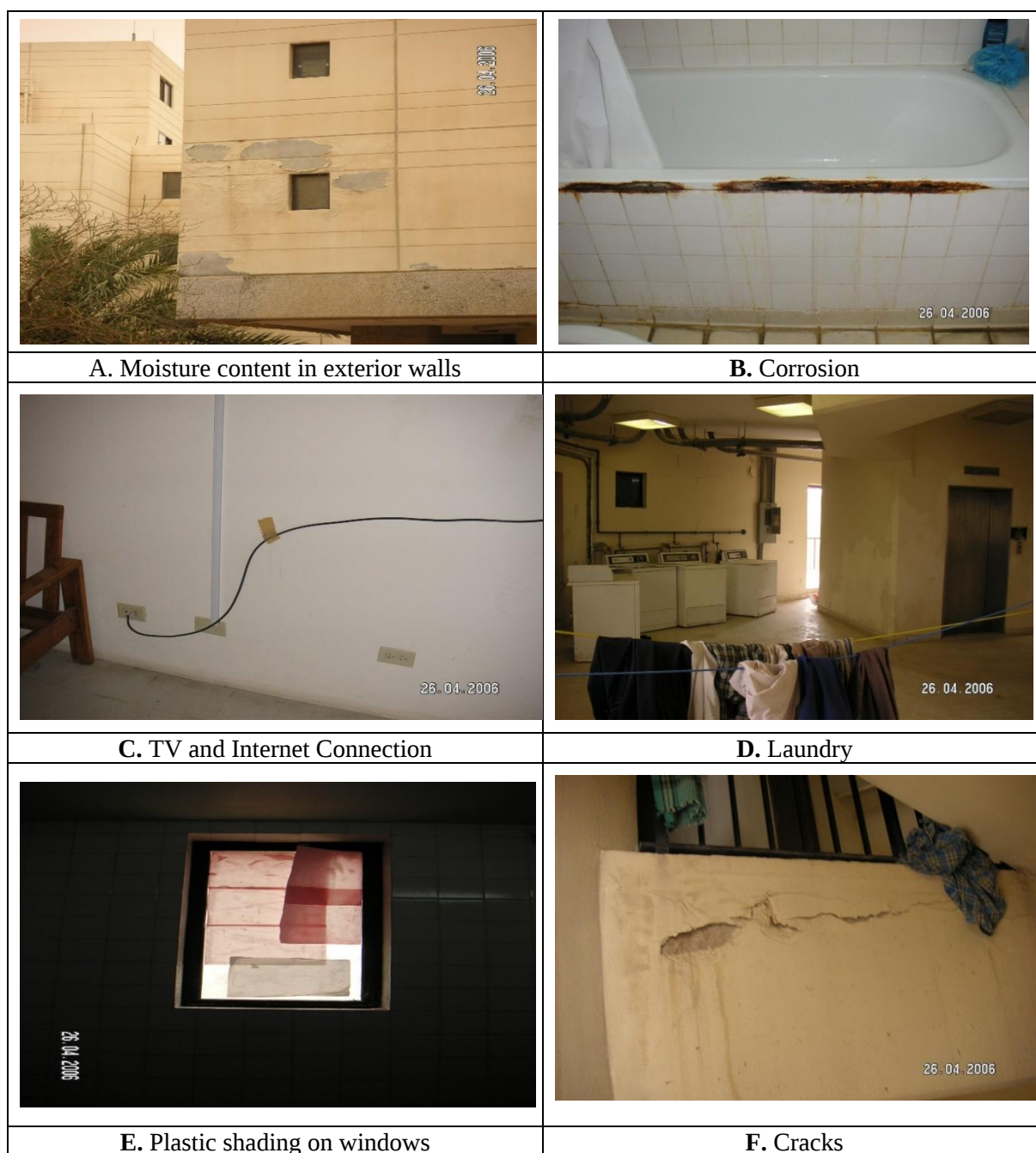
Figure 3 Photos show observed defects in the building.
